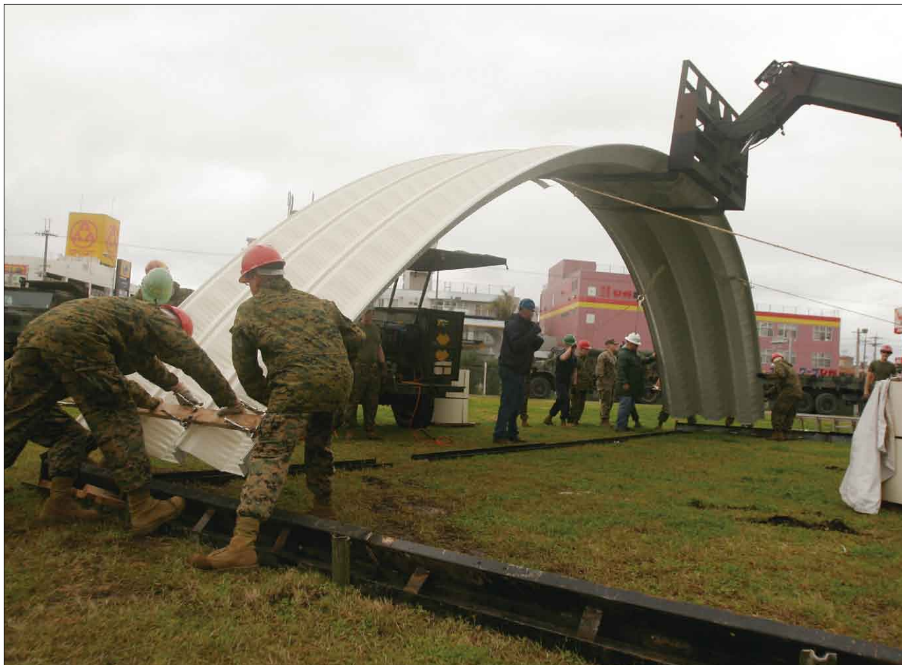
Combat engineers with Marine Wing Support Squadron 172 place panels created by the Ultimate Building Machine Feb 6. Photo by Lance Cpl. Corey A. Blodgett
