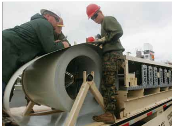
Keith Twing, a technical supervisor with MIC Industries (left), watches as Marines with Marine Wing Support Squadron 172's Combat Engineer Platoon prepare a coil of steel to insert into the Ultimate Building Machine.
